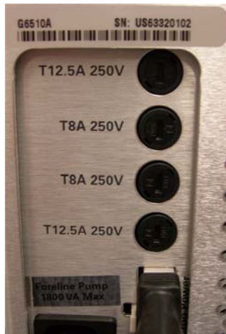
Figure 89 AC Board fuses
